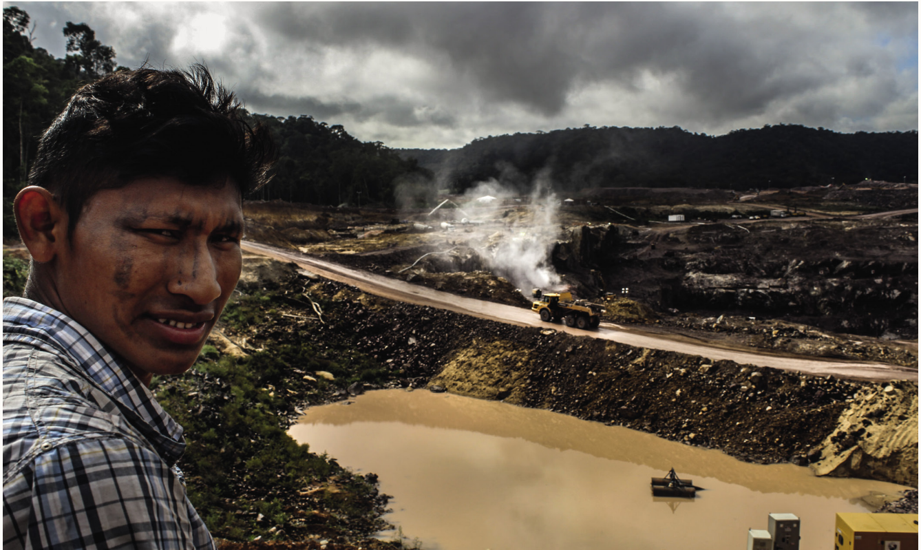
TELES PIRES RIVER | At the São Manoel Dam construction site on Brazil's Teles Pires River in 2015. Photo courtesy of Caio Mota/Forum.
