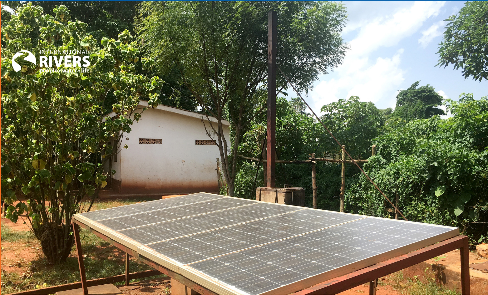
A health clinic located near the World Bank-financed Bujagali Dam in Uganda relies on solar power since the dam's power serves the capital, Kampala
