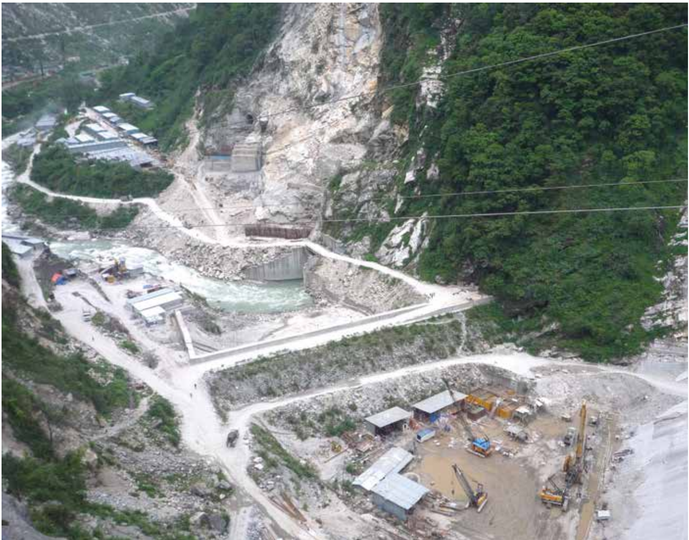
The under construction Teesta III Dam in Sikkim was affected by the earthquake in 2011. Photo credit: Samir Mehta
