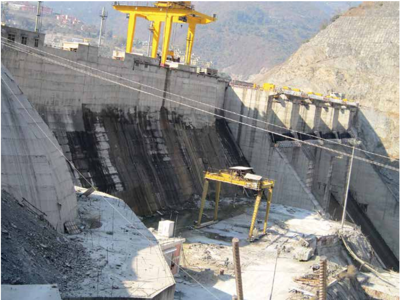
Koteshwer Hydroelectric Project on the Bhagirathiganga River, downstream of the Tehri Hydroelectric Project Photo courtesy: www.matuganga.blogspot.in
