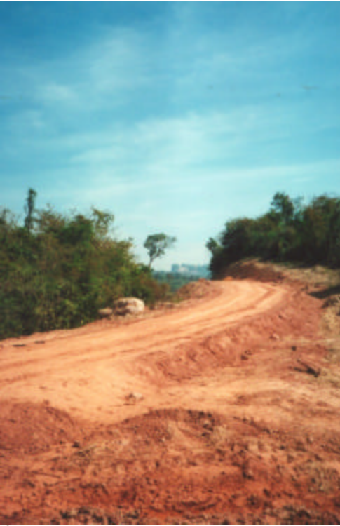
Construction of roads for the project will damage fragile ecosystems.
